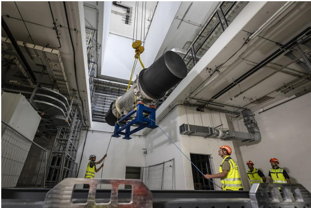
The installation of the FAIR accelerator machine has begun with the positioning of the first superconducting high-tech magnets (Image credit: GSI)
